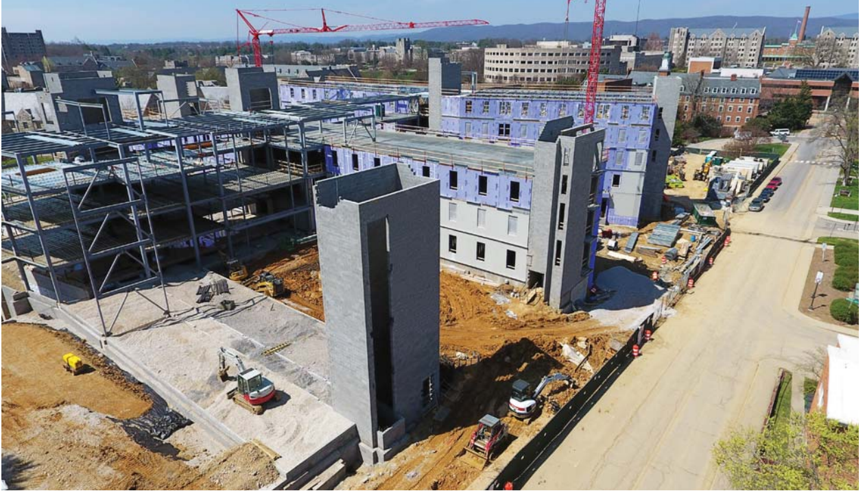
Early collaboration between a school and its design-build team can make all the difference in successfully constructing a building on a tight site in an established area on campus. Credit: W.M. Jordan
