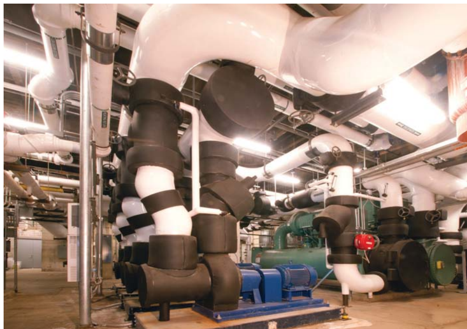
Butler University designed a new central chiller plant to support the growing campus, improve temperature control in existing facilities, and increase energy resiliency.
